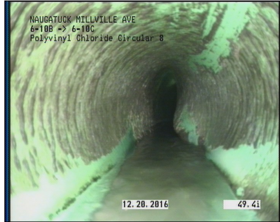
Photo: 53_6-10B_6-10C_20122016_D_D_48.44_131143.JPG, VCR No.: 57-122016-1, 00:00:00 48.44FT, Deformed, 55 %
