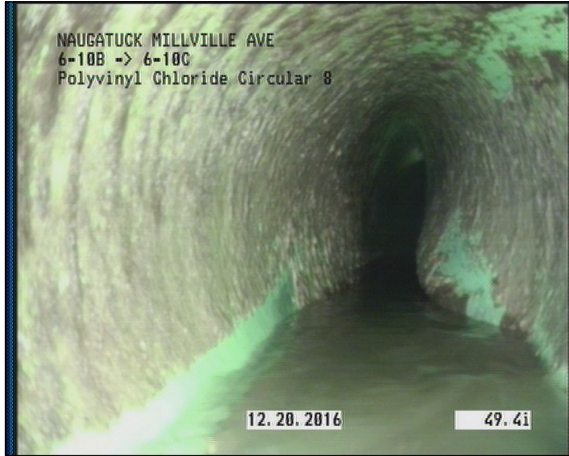
Photo: 53_6-10B_6-10C_20122016_D_D_48.44_131134.JPG, VCR No.: 57-122016-1, 00:00:00 48.44FT, Deformed, 55 %
