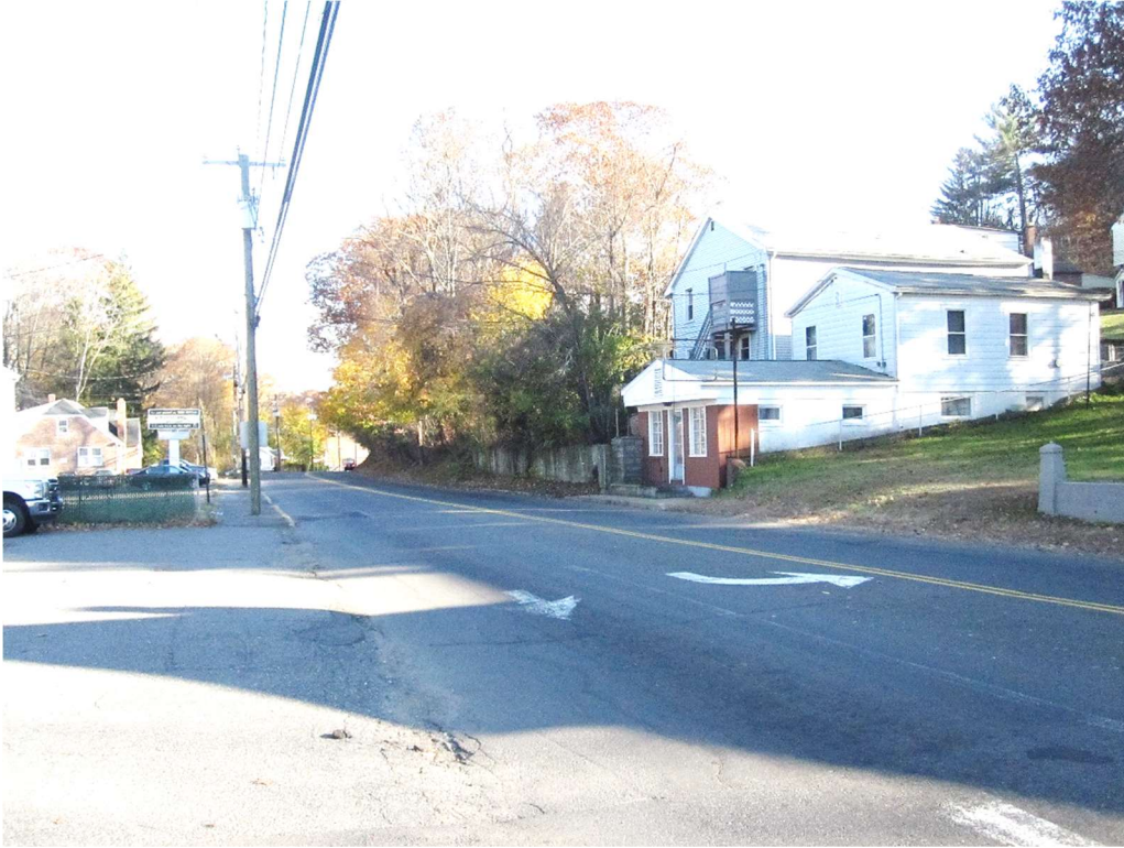
Photo 1. Pavement Condition – Rubber Ave. east of intersection with Melbourne Street, looking southeast
