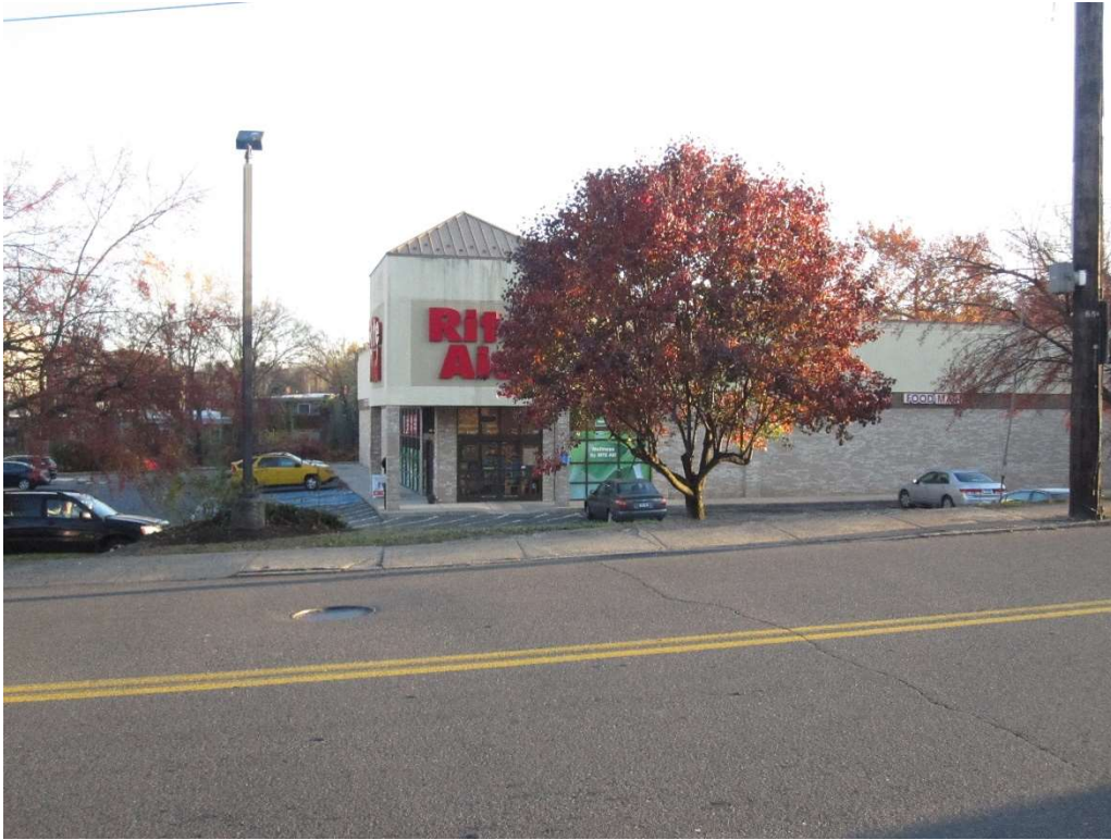
Photo 7. Pavement Condition – Rubber Ave. between Meadow St. and Church St.– Looking south
