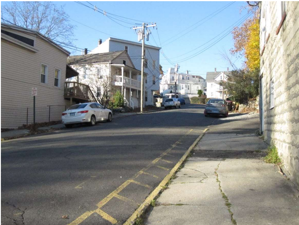
Photo 4. Pavement and Sidewalk Condition – Aetna St., looking north
