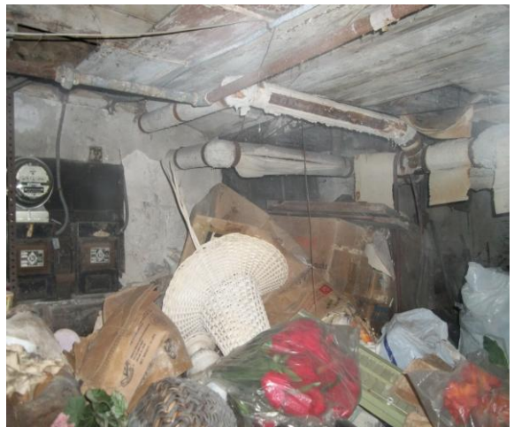
Photo #8 Damaged aircell insulation and stored materials in basement
