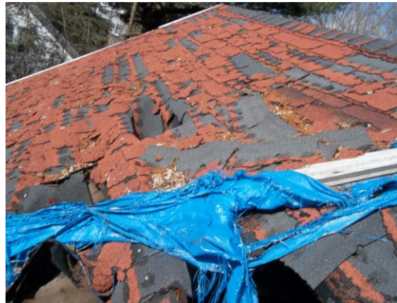
Photo #2: Holes in roof
