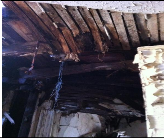
Photo #5: Collapsed ceiling joists
