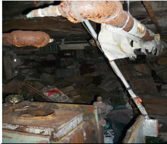
Photo #6 Damaged aircell insulation and stored materials in basement
