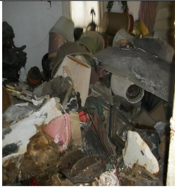
Photo #4: Stored items with collapsed ceiling debris
