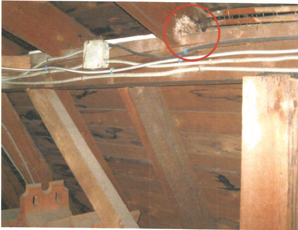
Water stained roof joist at bearing end
