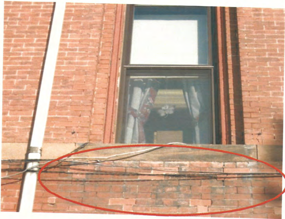
Failing masonry below window
