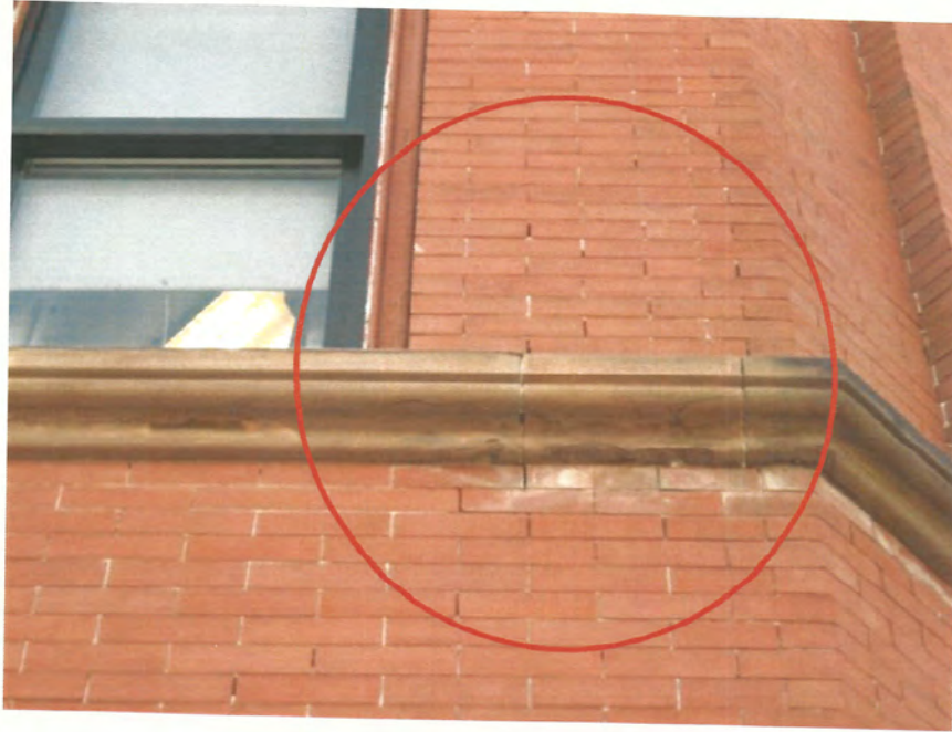
Voids in mortar joints
