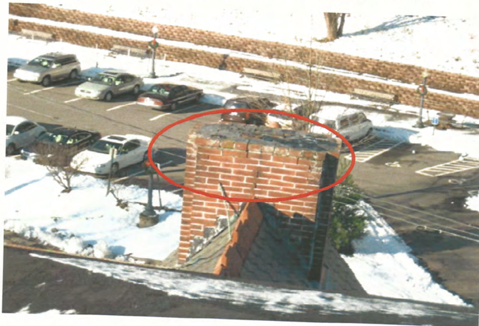
West chimney with spalling mortar and damaged brick
