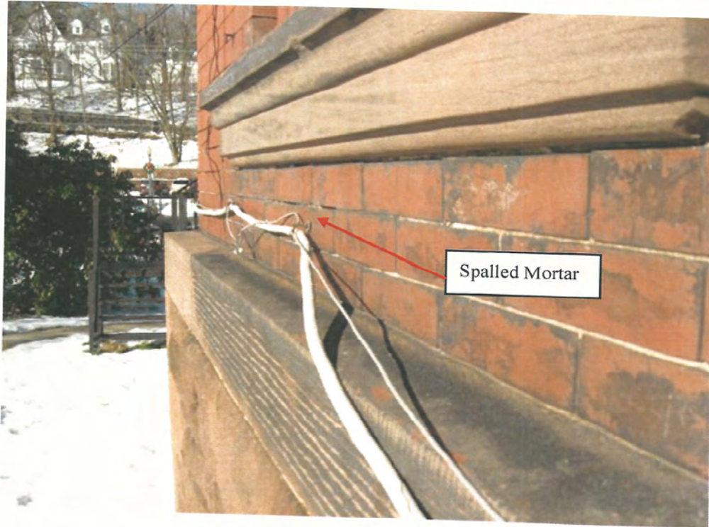
Spalling mortar joints in brick wall
