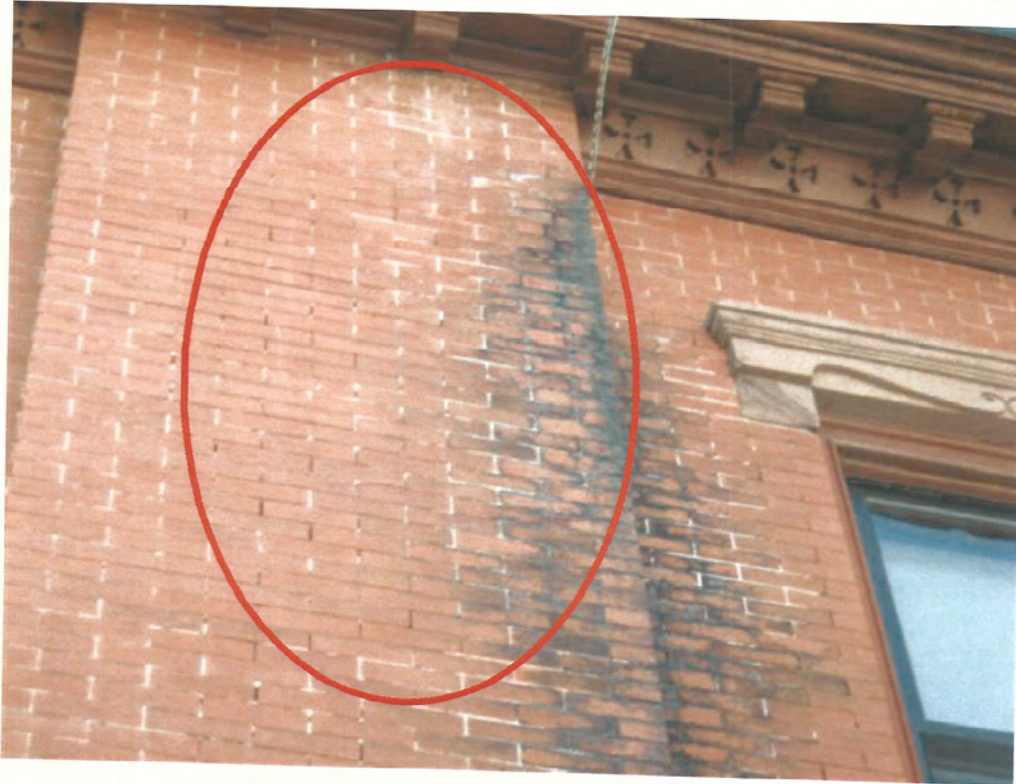
Voids in mortar joints and spalling mortar
