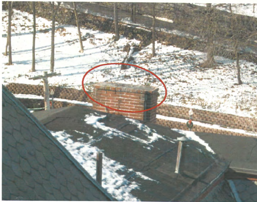
Missing Chimney Cap
