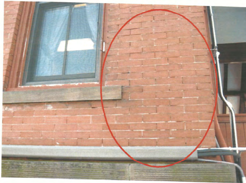
Voids in mortar joints
