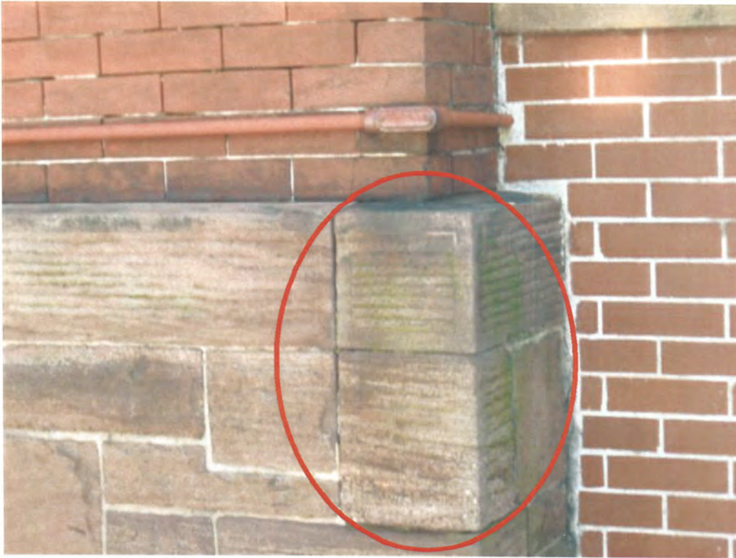
Spalled mortar in stone foundation wall and brick wall above
