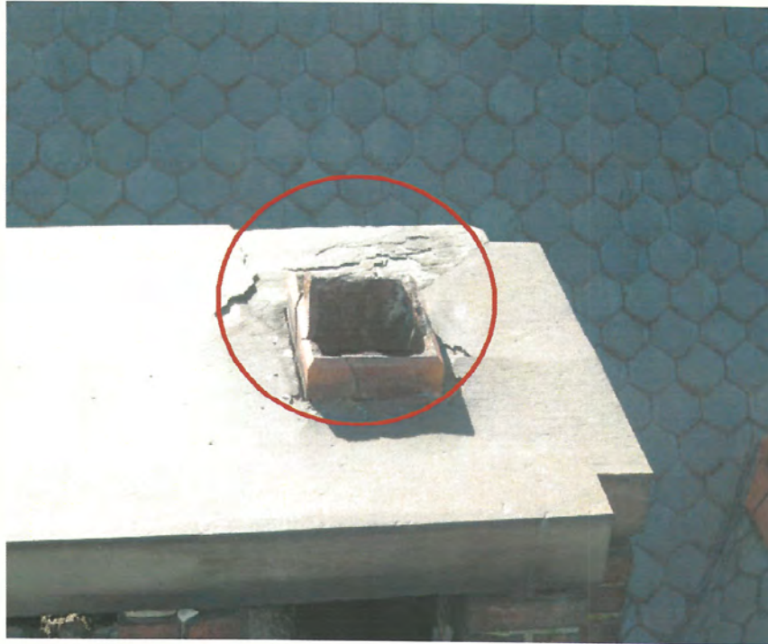
Damaged Chimney Cap
