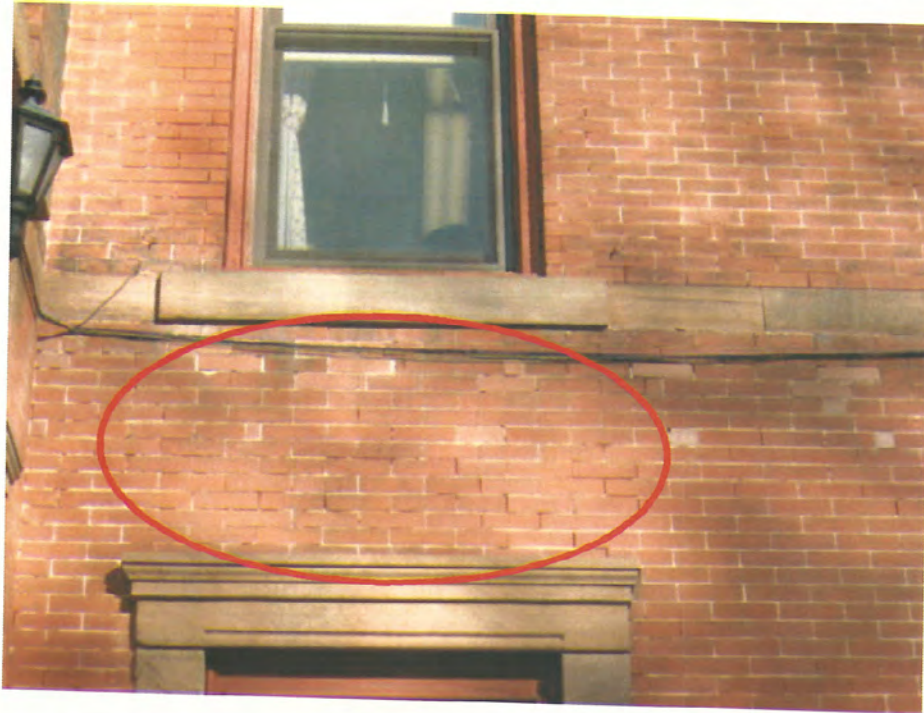
Movement above door opening with diagonal cracking
