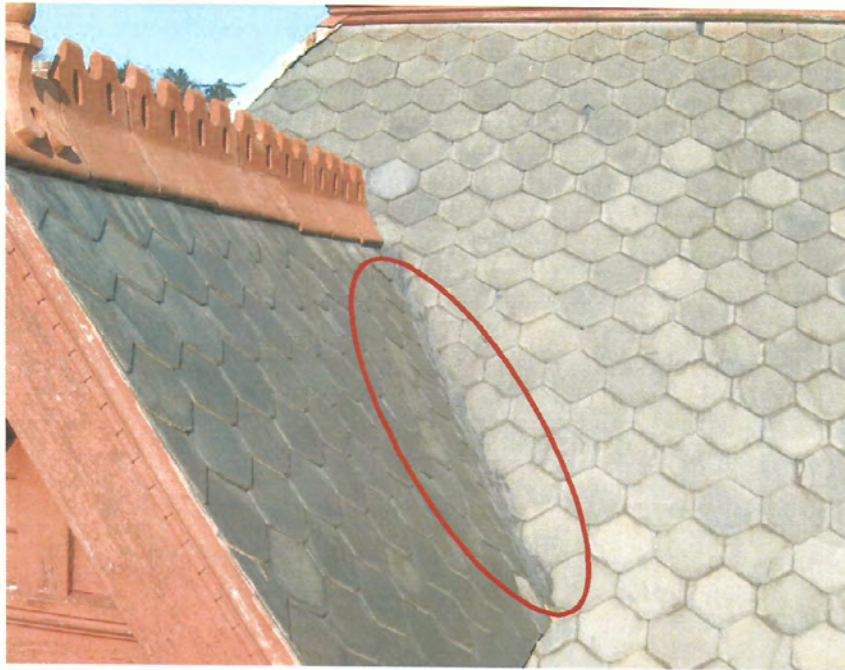
Copper Valley Flashing Covered with Roofing Cement
