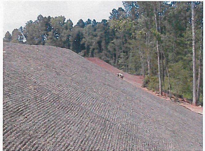
Example of Silt Fence Sedimentation Control
